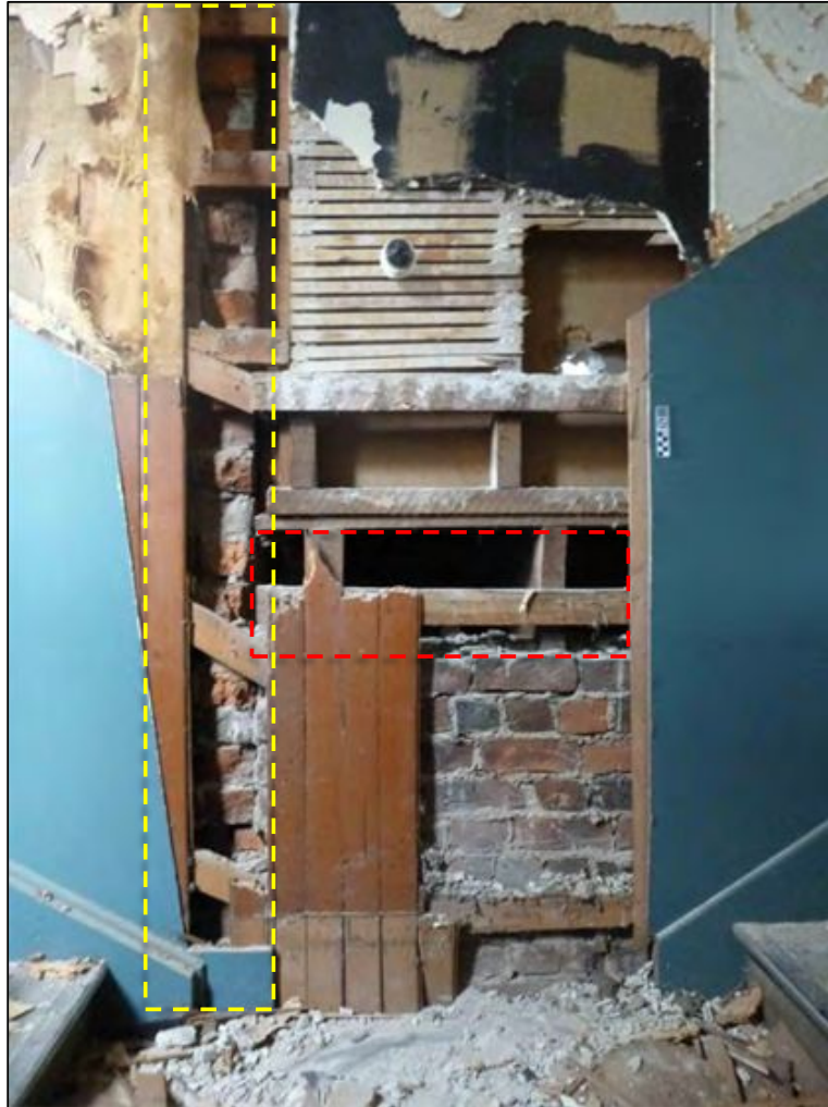
Figure 6-33 Sample area 10A showing join between original building and 1908 first floor extension, yellow dashed line outlines cut brick rear wall, red dashed line outlines the space between the ground floor ceiling and the first floor (photo faces east).
