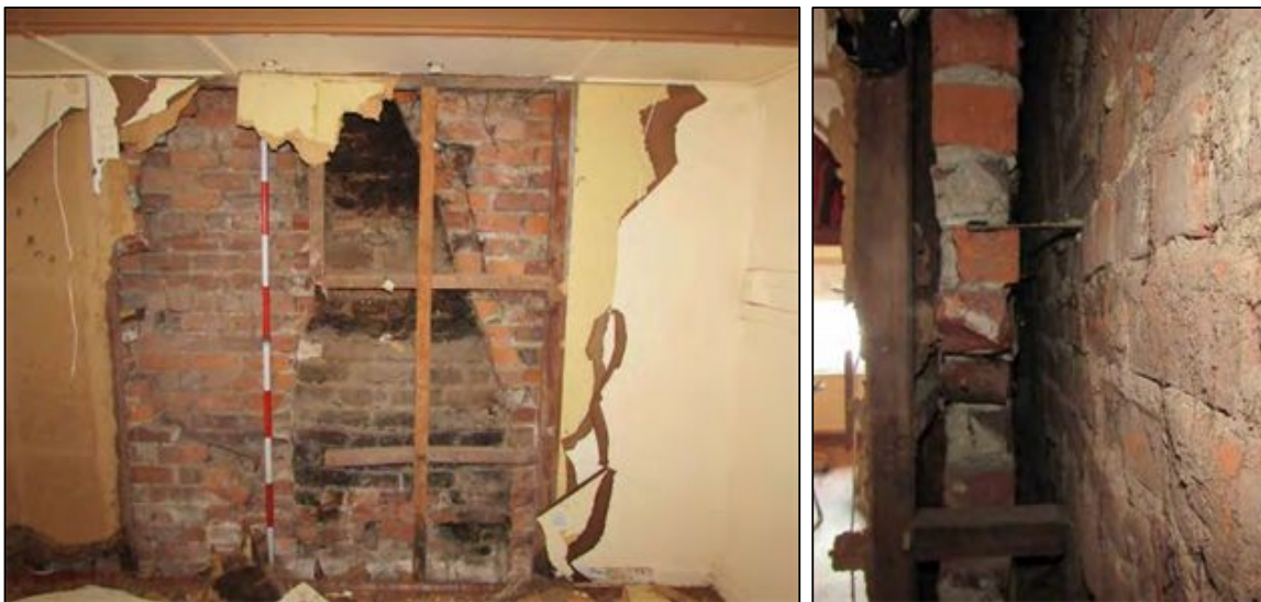
Figure 6-22. Left: photograph of the partially demolished fireplace and chimney on the west wall of Room 3. Right: photograph of the cavity wall between Rooms 3 and 23 (photo facing south).
