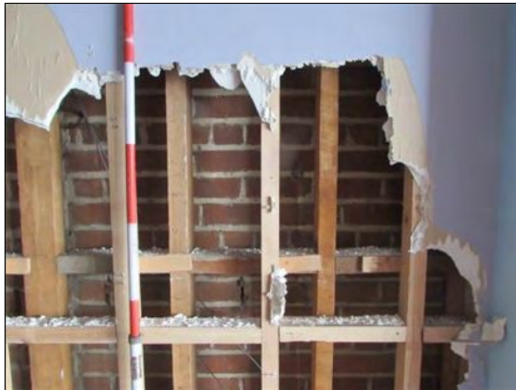
Figure 7-16. Photograph of sample Area 5A showing the original brick wall shared with the criterion behind two layers of timber framing (photo facing east).
