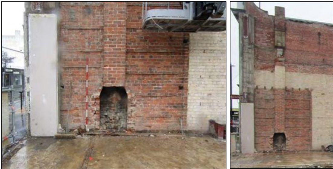
Figure 7-9. Right: brick fireplace and chimney in west wall of Rialto identified during demolition, scale is in 20cm increments. Left: photo showing full extent of fireplace and chimney with surrounding unpainted wall section (photos facing west).
