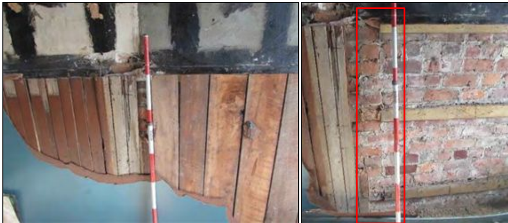
Figure 6-29. Photos of sample area 9B. Left: photo showing tongue-and-groove wainscoting and the sarking boards installed after the door was blocked. Right: photo showing edge of bricked up doorway outlined in red identified behind sarking boards (photos face east).
