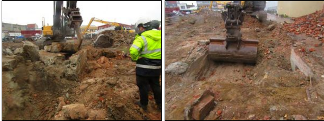
Figure 2-4 Area A removal of The Criterion Hotel foundations (left) and cellar excavation (right).
