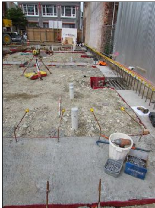
Figure 2-12 Trench for drainage, Area AD, filled in and marked by grey protruding pipes, photo faces south.
