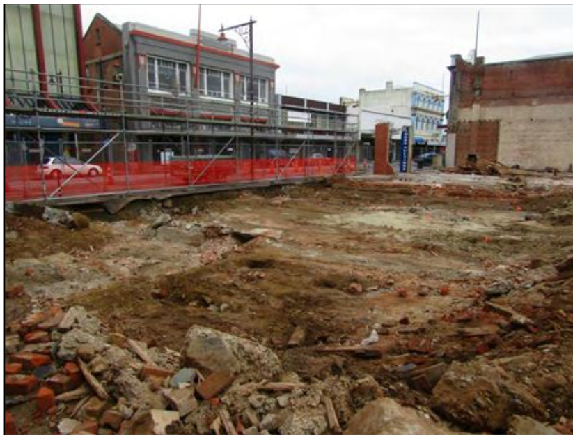
Figure 6-67. Photo of Excavation Area A showing natural topsoil exposed below the buildings footprint and patches of demolition rubble in the foreground. Photo faces south-west.
