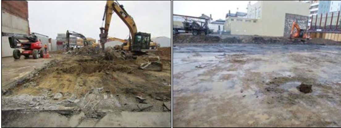
Figure 2-9 Removal of building foundations Area B (left) and site clearance Area E (right)
