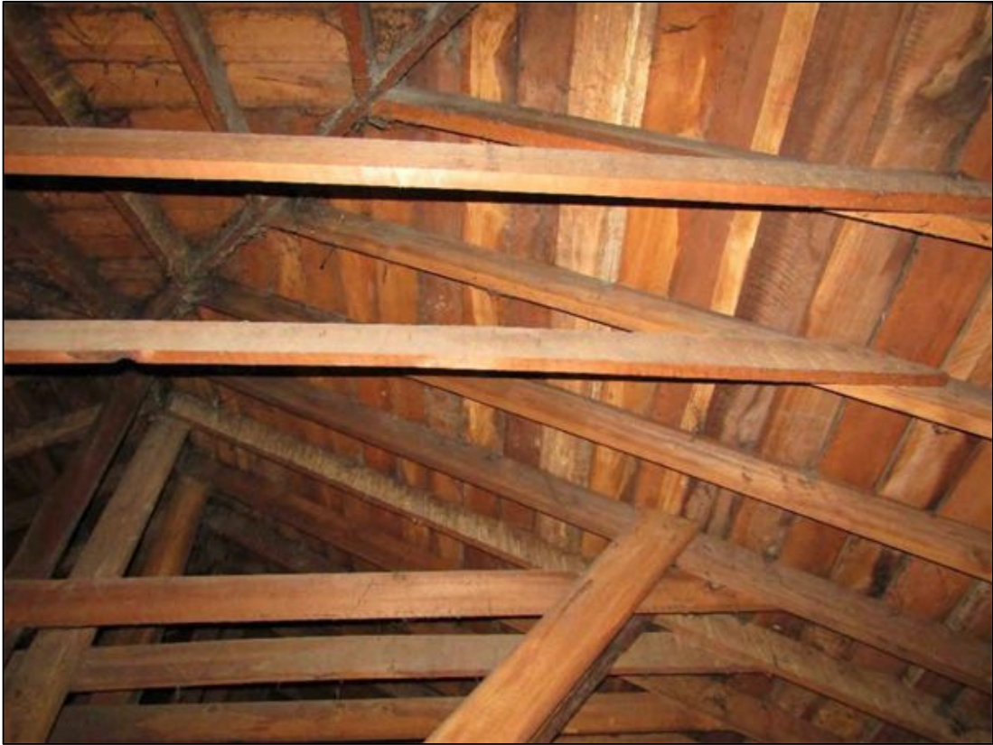
Figure 6-15. Roof space above original building showing sarking board cladding and roof structure (photo faces up and west from roof access in Room 15).
