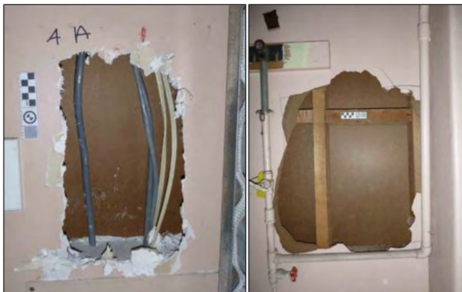
Figure 7-14. Left: sample Area 4A showing plasterboard lining (photo facing east), Right: sample Area 4B showing hardboard lining and timber framing (photo facing west).
