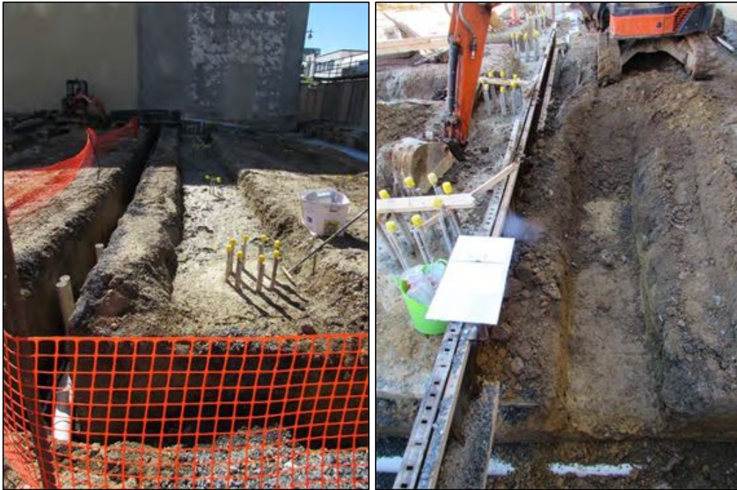
Figure 2-7 Excavation of drainage trench Area AD, note drainage trench on left and line 8 on right (left) and drainage trench being excavated in centre and line F on left (right)
