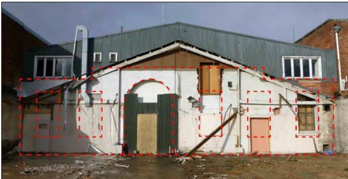
Figure 7-5. Photo of the rear wall of the Rialto red dashed lines indicate the original shape of the structure and window and arched access way locations (photo facing south).
