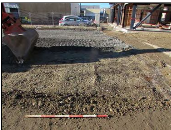
Figure 2-3. Site scraping at south end of Area AR for carpark. Photo faces east.
