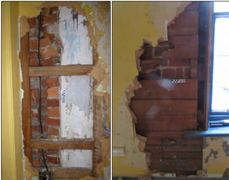
Figure 6-50. Left: photo of sample area 22A showing plaster coat of north wall and cross section of original west wall. Right: photo of sample area 22B showing sarking and brick wall partially exposed (photos face north).
