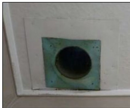
Figure 6-46. Photo of chimney flue and firestop with metal cover removed in north-west corner of Room 19.
