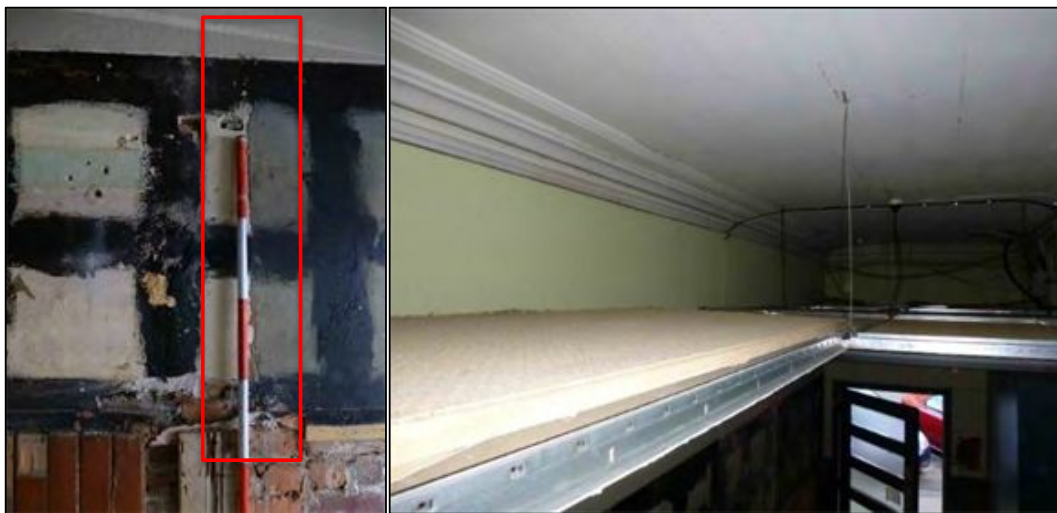
Figure 6-30. Left: Photo of sample area 9B showing plaster coat and fine concrete coat transition outlined in red (photo faces east). Right: Photo of space above dropped ceiling showing period style cornice in place and tongue-and-groove ceiling (photo faces south east).
