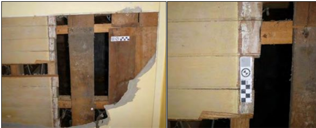
Figure 6-52. Left: photo of sample area 22D showing exposed tongue-and-groove, and sarking ceiling linings. Right: photo of tongue-and-groove lining showing edge of paint (east is to the left).
