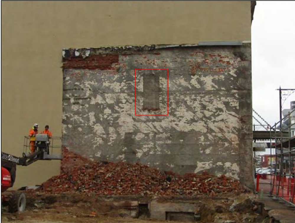
Figure 6-37. Photo showing window cavity identified in Room 13 during demolition. Photo facing east.
