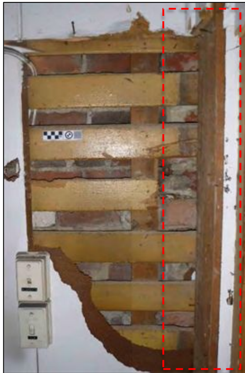
Figure 6-58. Photo of sample area 23C showing tongue-and-groove boards behind hardboard lining, remnants of previous brick wall outlined in red (photo faces west).
