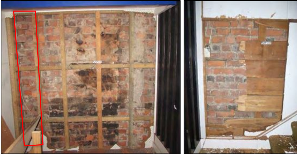
Figure 6-54. Left: photo of the partially demolished fireplace and chimney on the west wall of Room 23, remnants of removed brick wall outlined in red. Right: photo of the west brick wall exposed behind the wider sarking boards to the north of the fireplace.
