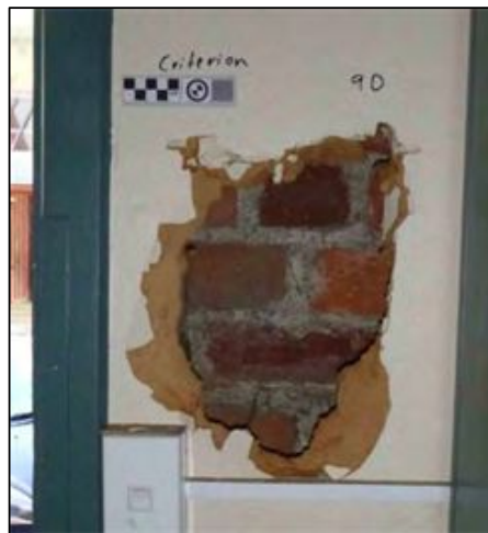
Figure 6-28. Photo of sample area 9D showing brick wall behind modern linings (Photo faces south).
