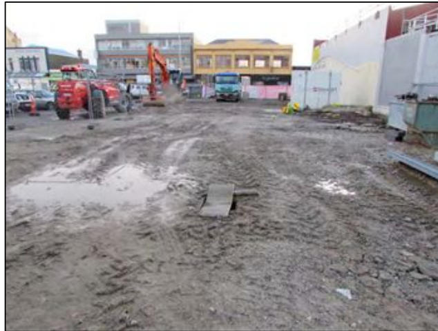
Figure 5-4. Excavation Area AR prior to scrape. Context AR3 covers the site. Photo faces north.
