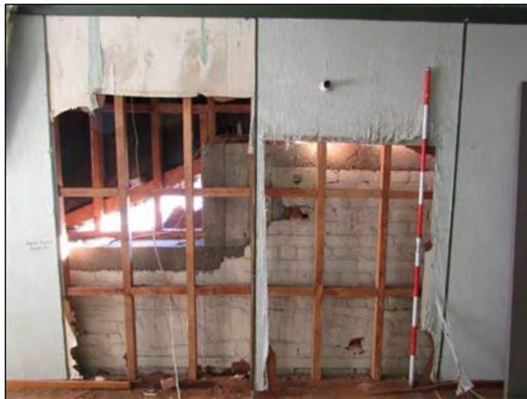
Figure 7-18. Photograph of sample Area 11A showing the modern stud wall in front of the original north brick exterior wall with modern timber framing on top, brick relieving arch and lintel are visible at the bottom of the image (photo facing north).
