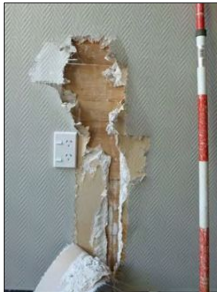
Figure 6-36. Photo of sample area 11A showing modern timber wall exposed behind plasterboard lining (photo facing west).
