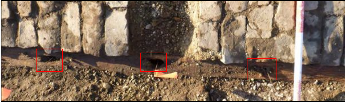
Figure 6-71. Detail of three of the notches identified in the wooden beam/bottom plate (F28).
