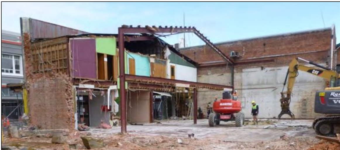
Figure 7-7. Photograph of the Rialto building during demolition showing the exposed steel frame, partially demolished eastern brick wall and intact west brick wall (photo facing south-west).
