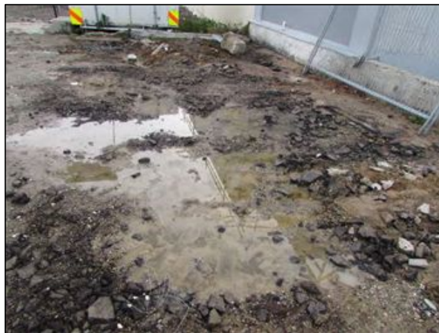
Figure 5-5. Excavation Area AR prior to scrape. Photo shows asphalt of Context AR2. Photo faces north.
