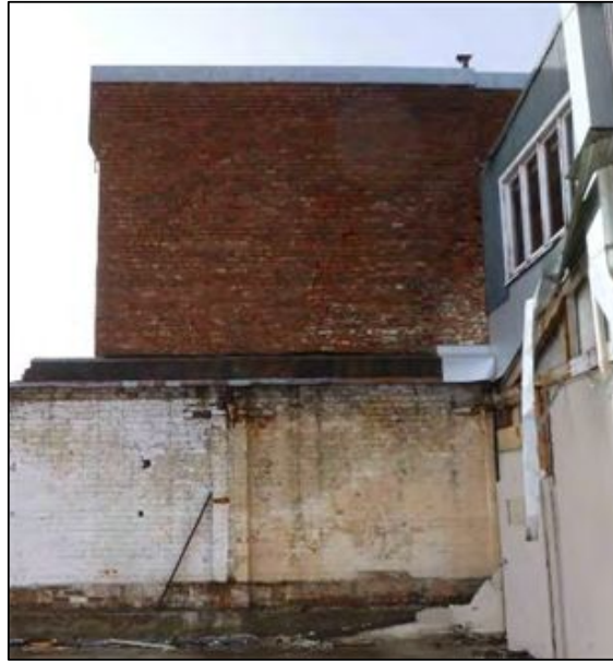
Figure 6-11. Photo of the west façade of the rear section, white painted bricks are part of the neighbouring building which has been mostly demolished.
