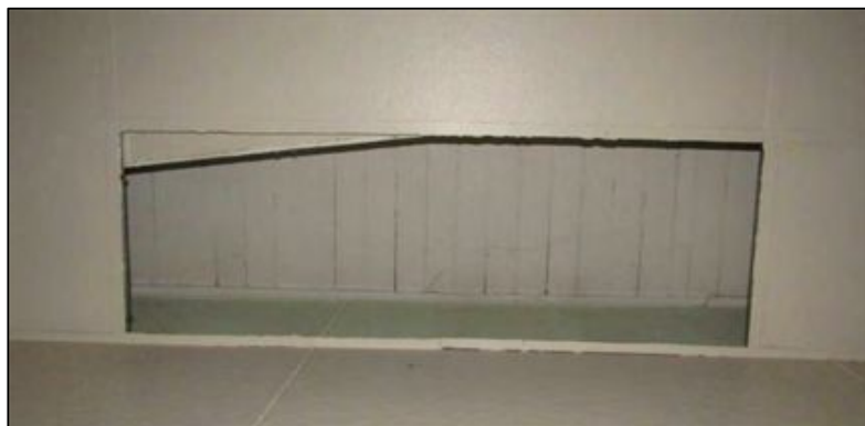
Figure 6-34. Sample area 10B showing tongue-and-groove ceiling above modern dropped ceiling (north is to left).
