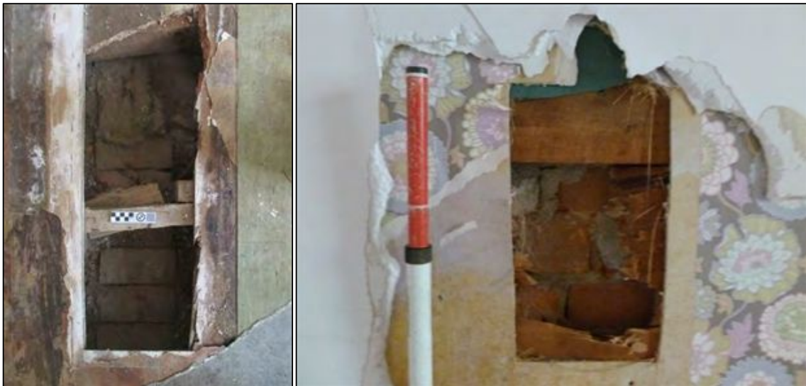
Figure 6-25. Left: photo of sample area 8A showing row of bricks below tongue-and-groove floorboards (north is to the top of the photograph). Right: photo of sample area 8B in north wall showing brick wall below various layers of linings.
