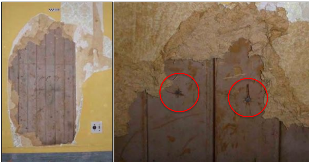
Figure 6-51. Left: photo of sample area 22C showing tongue-and-groove panels behind modern softboard. Right: close-up of nails with remnants of scrim circled in red (photos face south).
