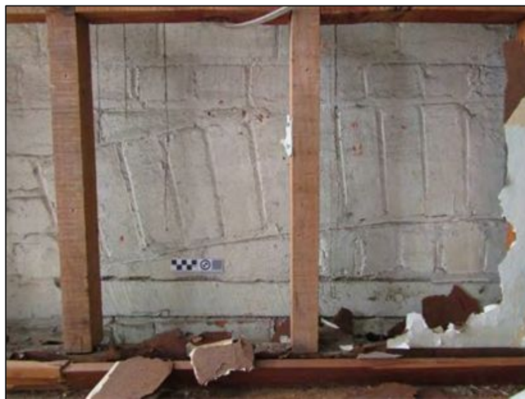
Figure 7-19. Detail of relieving arch and lintel in north wall (photo facing north).
