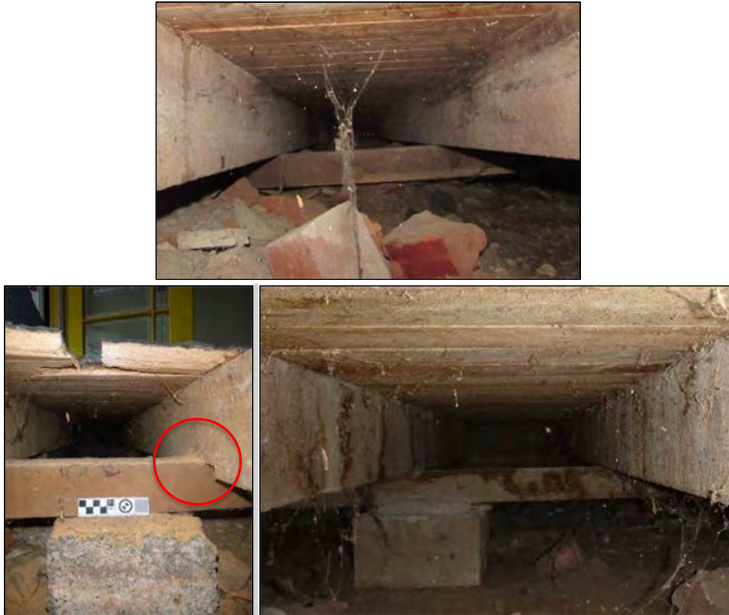
Figure 6-14. Top: Photo of subfloor in original building (Room 3) (photo faces north). Bottom Left: Photo of subfloor in 1894 extension showing notched joists circled in red (photo faces west). Bottom Right: Photo of subfloor in 1908 extension (Room 8) (photo faces west).
