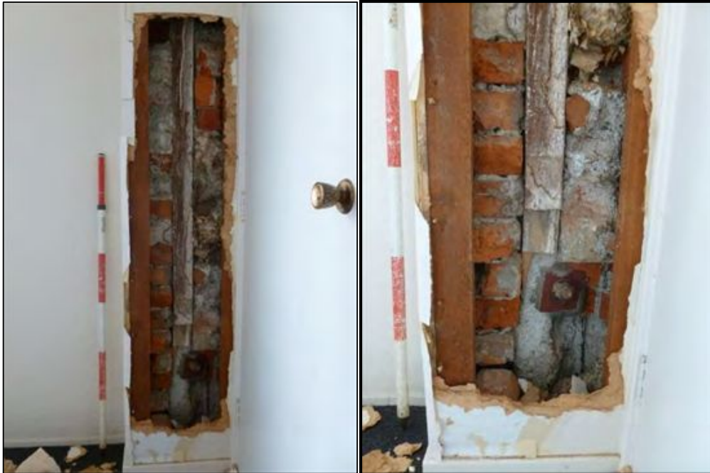
Figure 6-45. Photos of sample area 19A showing the remains of the original exterior wall of the hotel (photos facing south).
