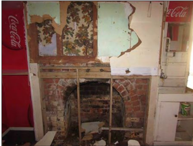
Figure 6-19. Brick fireplace exposed beneath several layers of modern linings in Room 2 of the Criterion Hotel.
