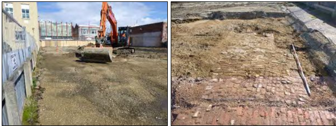
Figure 2-5 Beginning of site clearance in Area F, looking south (left) and exposing brick floor in Area F, looking north (right).
