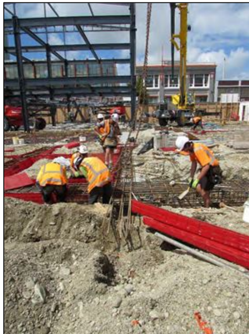
Figure 2-8 Site showing imported shingle surface and shallow excavations required for some foundation lines. Area AO (line D) in centre of photo, facing south.
