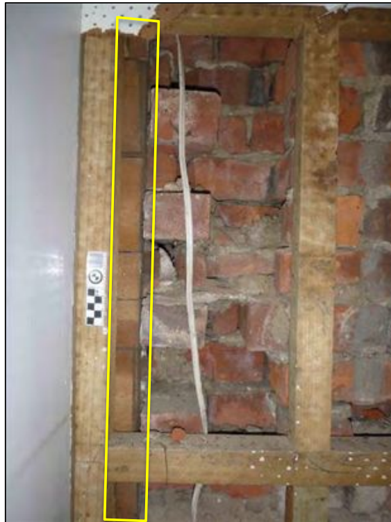
Figure 6-55. Close-up photo of the remnants of the removed brick wall, the ends of the sarking boards can be seen to the left out lined in yellow (photo faces west).
