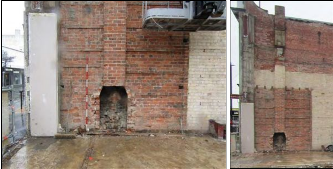
Figure 7-47. Right: brick fireplace and chimney in west wall of Rialto identified during demolition, scale is in 20cm increments. Left: photo showing full extent of fireplace and chimney with surrounding unpainted wall section (photos facing west).
