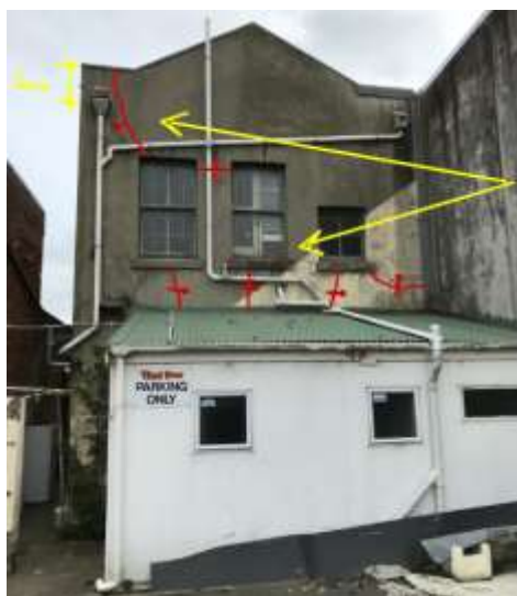
Photo 1: Rear of building showing lines of cracking.
