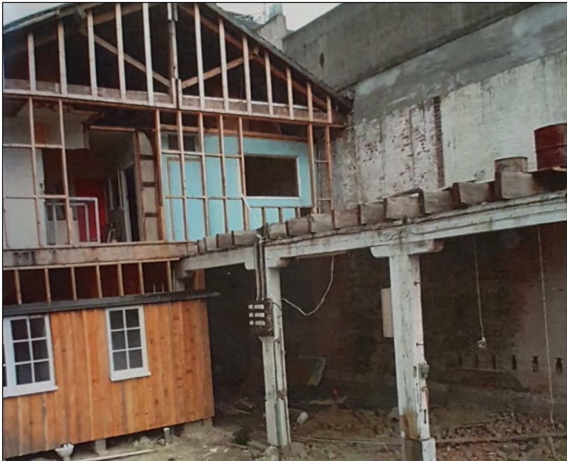
Figure 4-25. Detail from 2004 image taken by the ICC showing demolition of rear portion of 12-14 Esk Street in progress (ICC Property File).
