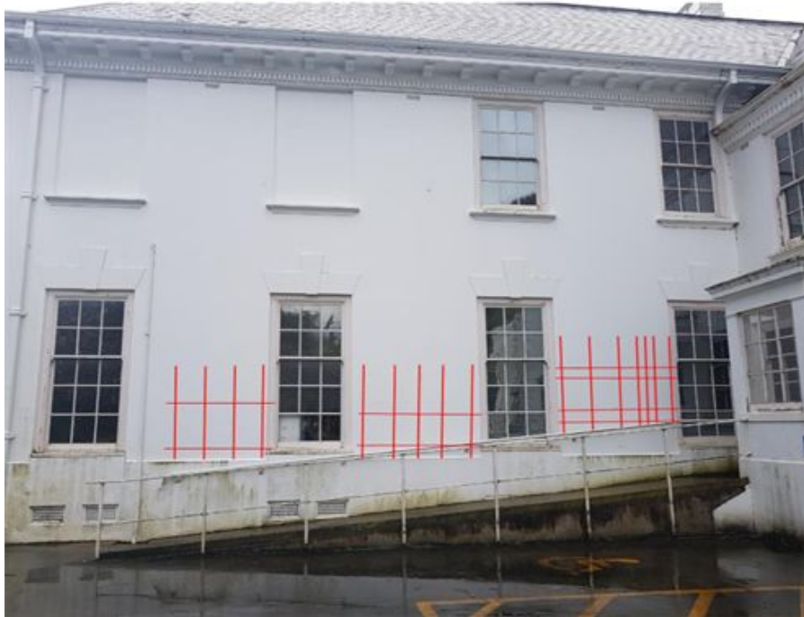
Figure 1: Approximate steel reinforcing in concrete veneer which was identified during the site inspection
