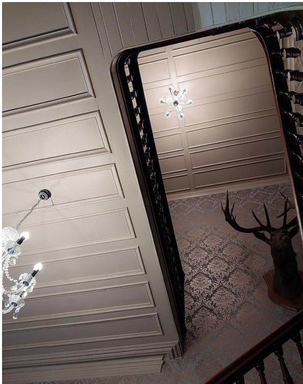
Figure 5 – The first storey stairwell ceiling now matches the ground floor ceiling (original)
