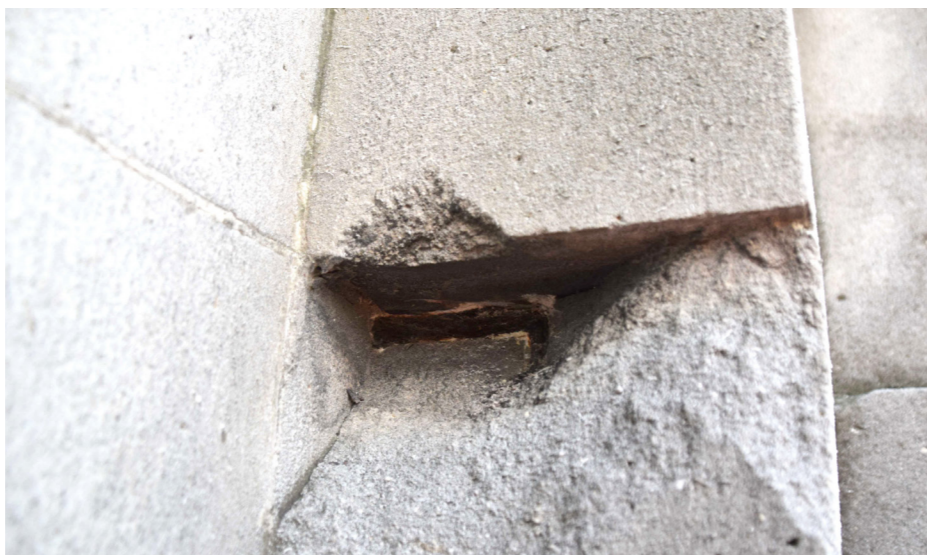
An iron cramp embedded in the stonework, corroded and expanded over time, causing stonework to crack and fall away
