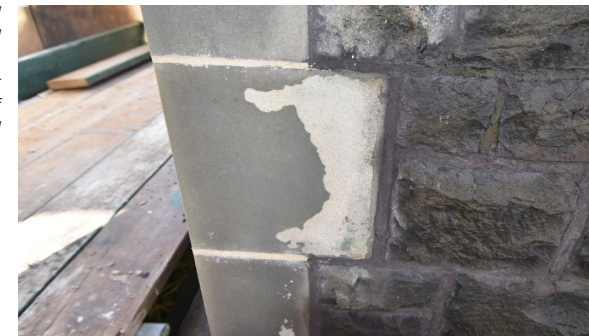
A previously applied sealant has attracted pollution on the quoin, forming a dark skin that is no longer capable of being cleaned
