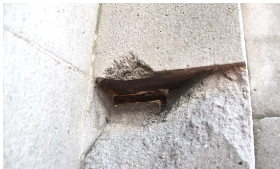
An iron cramp embedded in the stonework, corroded and expanded over time, causing stonework to crack and fall away
