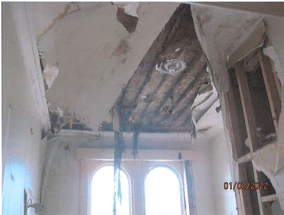
Typical water damage to ceilings, timber work and walls at first floor level. Other linings damaged by vandalism to the right of the photo
