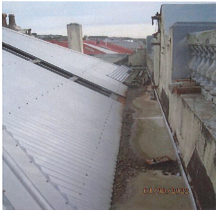
Similar view further to the west end, gutter corroded out and roof sheeting missing and open though to floor below. No cover flashing to gutter edges behind wall and open to below
