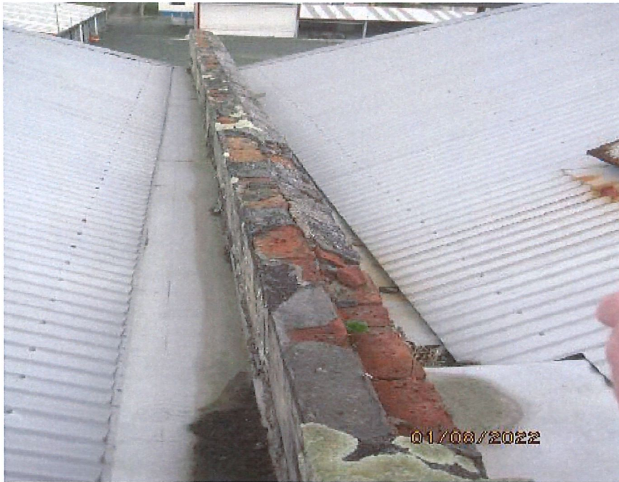
Typical view of poor condition to top of parapets of original intertenancy walls showing open brickwork and joints allowing water to track inside the walls.
