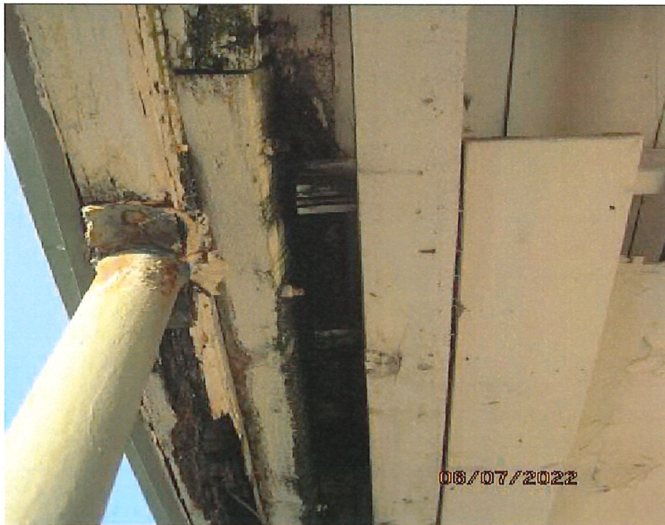
View of a similar post in poor condition and badly rotten beam above
