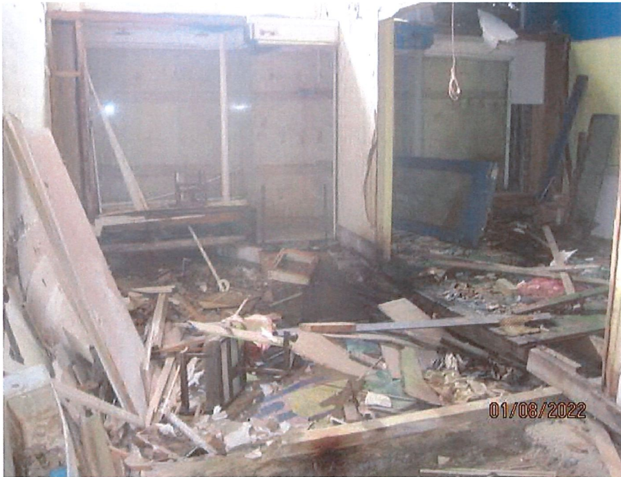
Typical damage from vandalism to ground floor area, actual flooring has been removed. Area is being saturated from water entering above first floor
