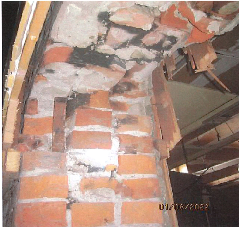
Condition of a brick opening punched through a ground floor masonry wall. No lintel or trimming frame to support wall loads from above. note areas of fire damaged brick from original fire in 1914.
