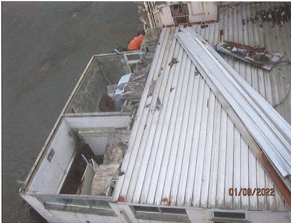
Rear view of site showing single storey block masonry extension and roof partially demolished.
