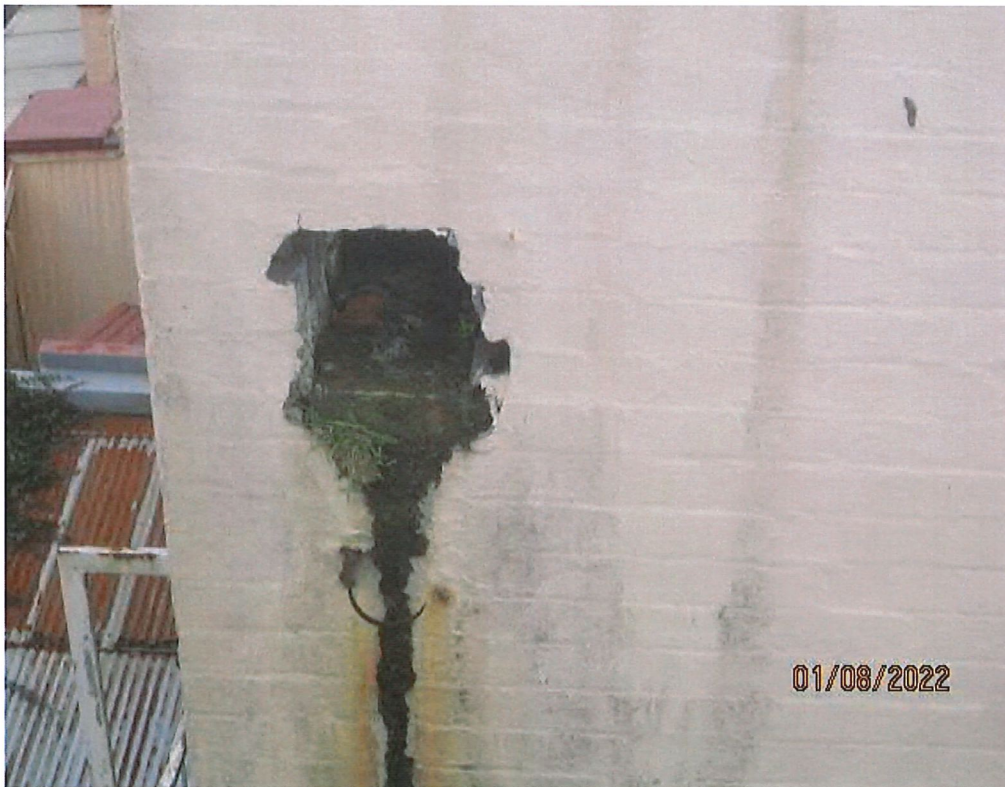
Missing gutter extension, rainhead and downpipes allowing water to flow back inside the building and also directly into the brick work layers.
