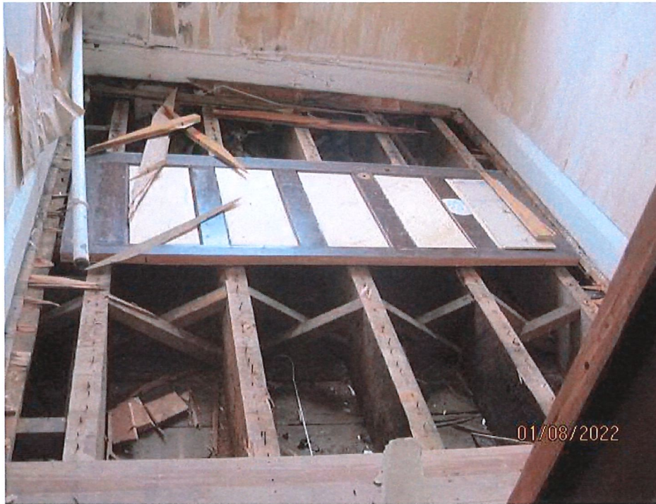
Flooring removed at first floor level typical in many rooms. Typically there is no physical connection between the floor joists and the exterior brick walls to restrain the walls
