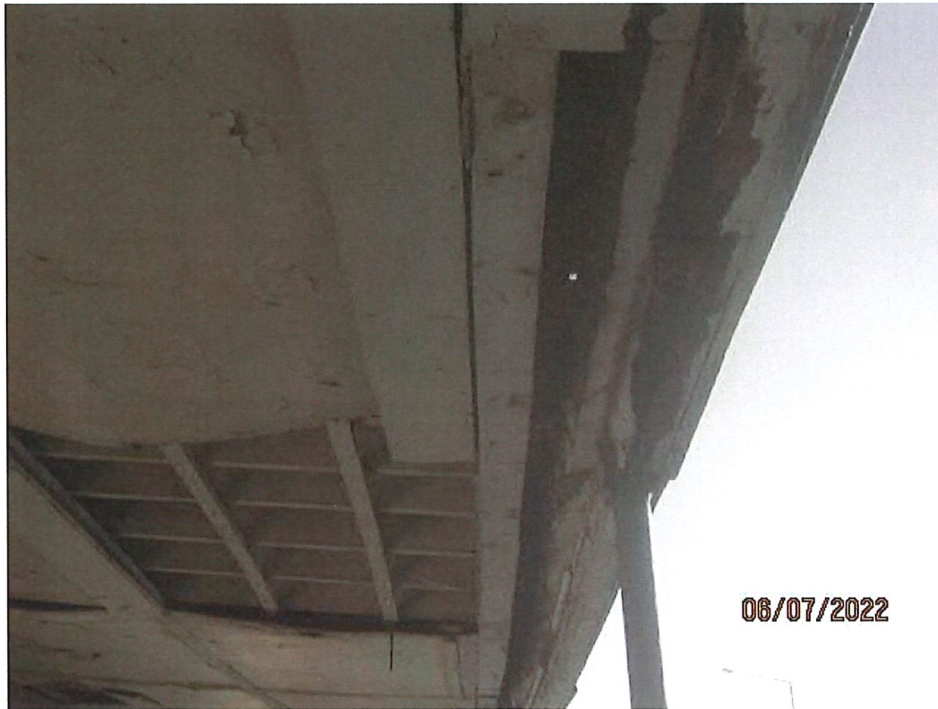
Water damage to soffit linings and outer main support beam in very condition also. Very poor condition to all nail fixings
