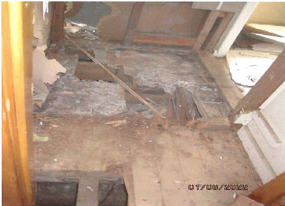
Typical view of upper floor area damage to floors and wall linings.
