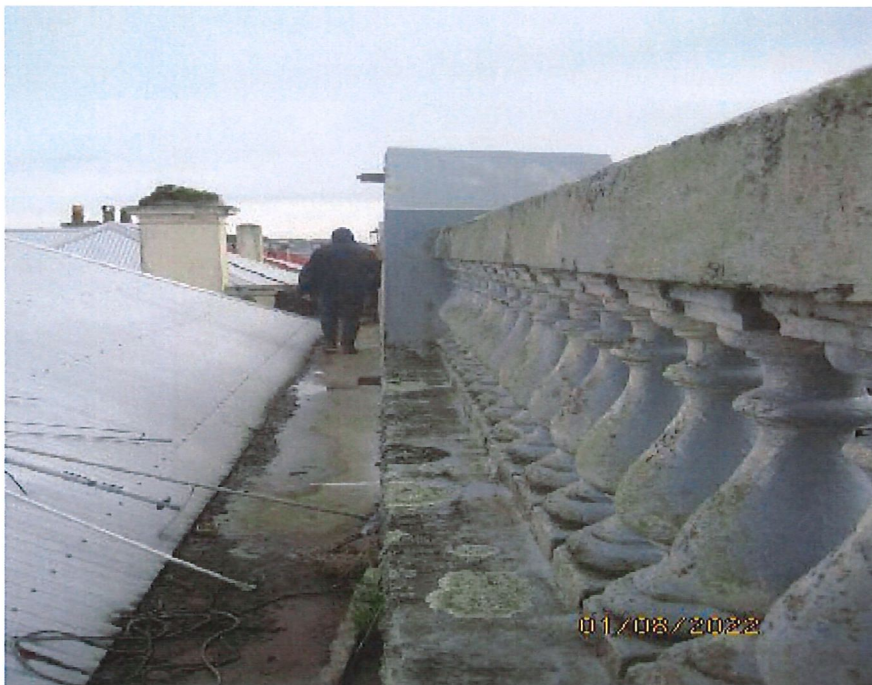
View behind main façade at roof level, the heavy parapet is leaning out approximately 75mm.
