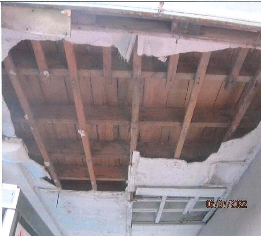
Closeup view of damaged and collapsed soffit lining showing typical construction
