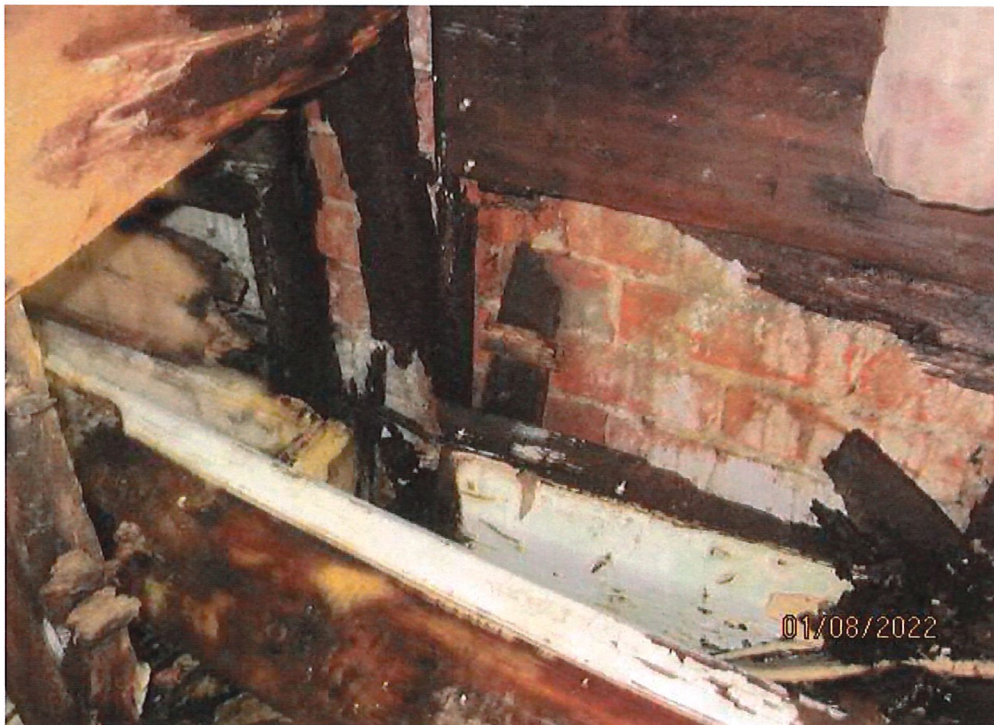
Water damaged and rotten timber wall framing to exterior wall, flooring and wall linings have also rotted away
