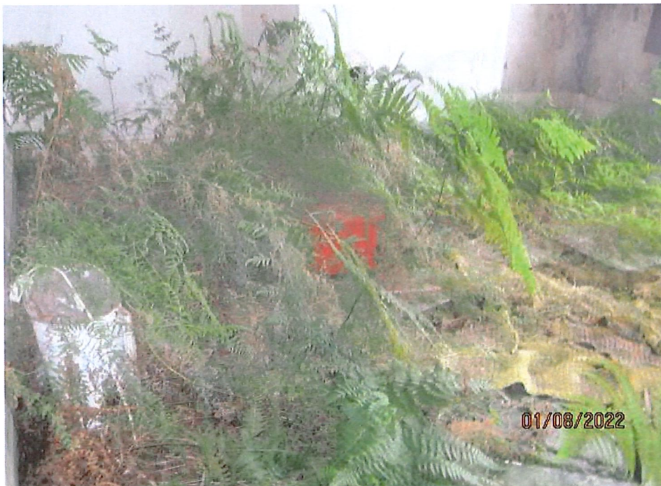
Additional view to rest of the same room showing even heavier buildup of vegetation. There is black mould on the walls also
