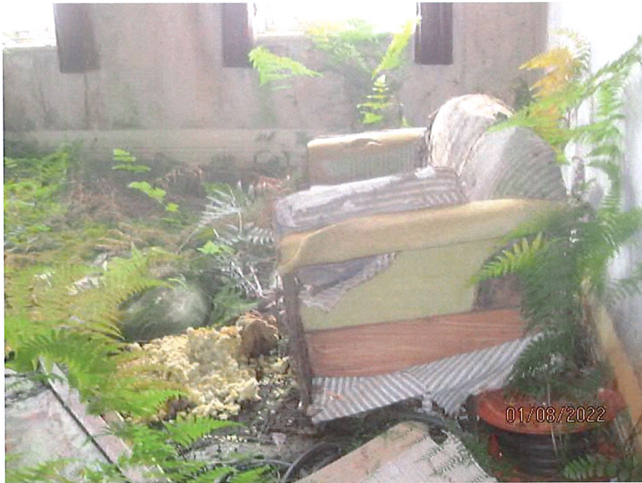
Extent of water damage over time and buildup of vegetation in one of the rooms. Room was deemed to be dangerous to enter
