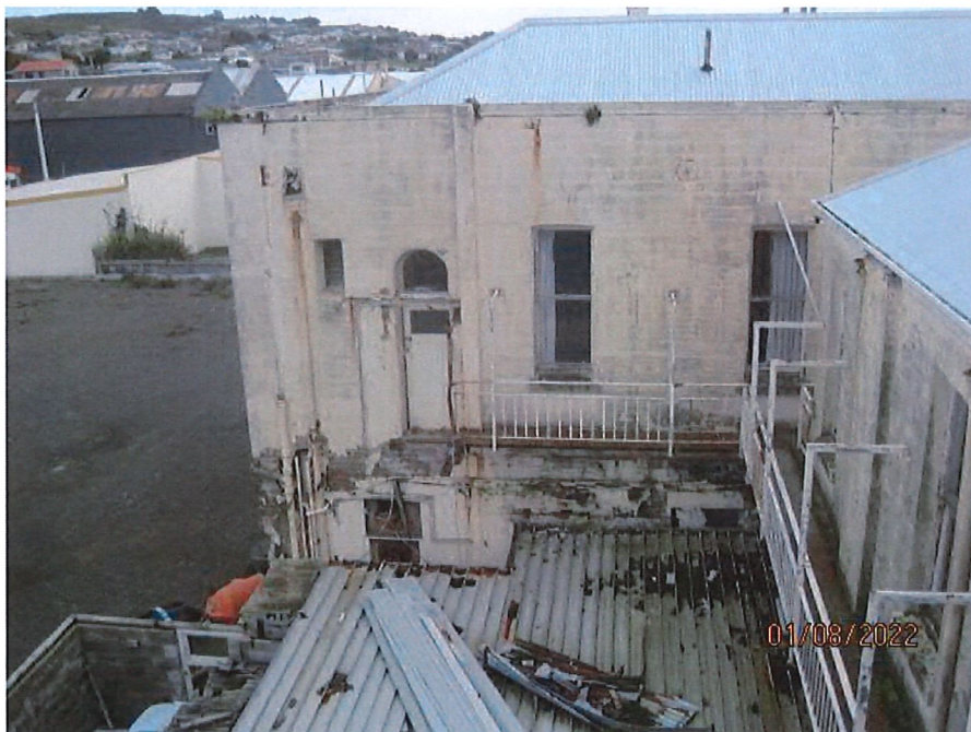
View to rear of the building, with partially demolished roof to lower left Cantilevered fire escapes attached to buildings
