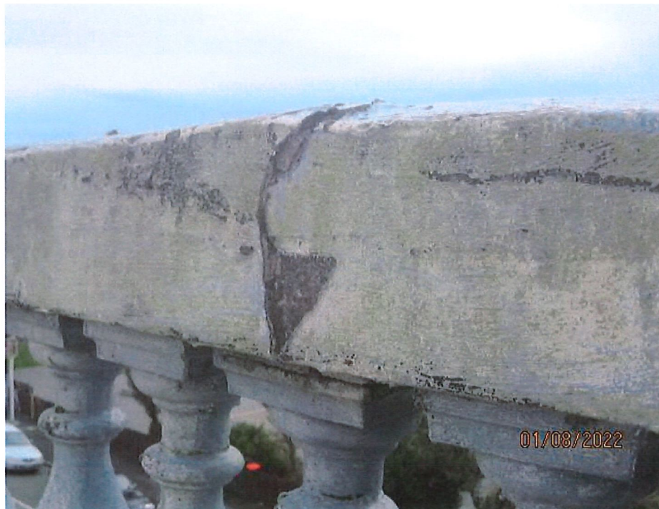
Typical condition of capping beam over pedestals showing crack and slight offset out towards the street.
