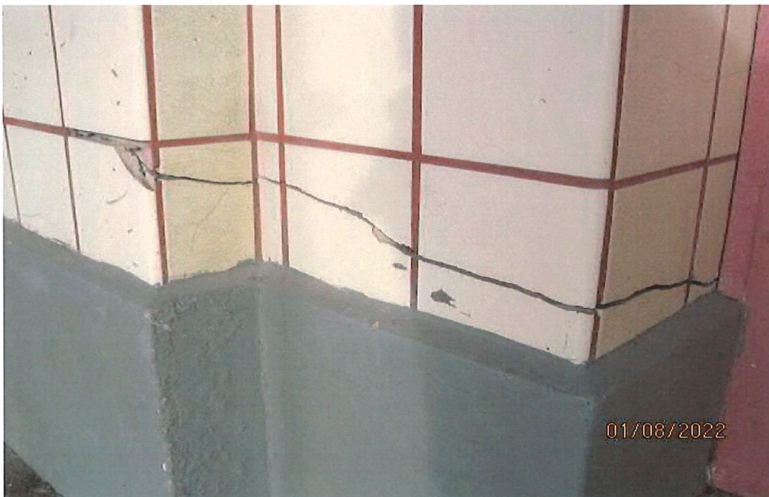
Large open tension crack visible to the base of the column by ground floor main entry door
