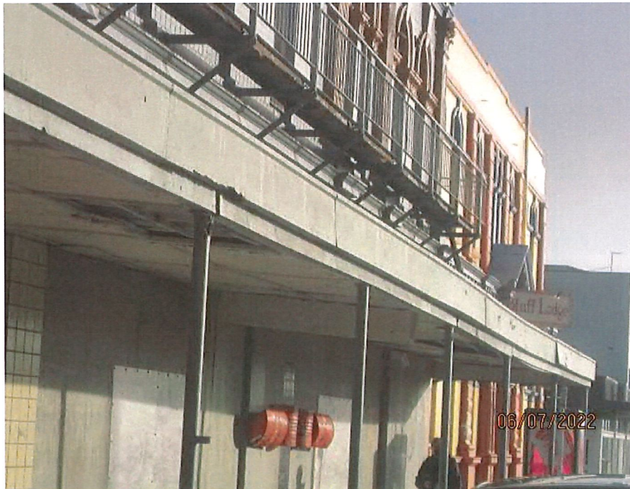
View along front façade showing veranda in very poor condition and the corroded fire escape above.
