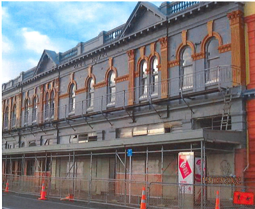
View of ornate front façade with veranda cordoned off, Note heavy parapet and cornice at roof level
