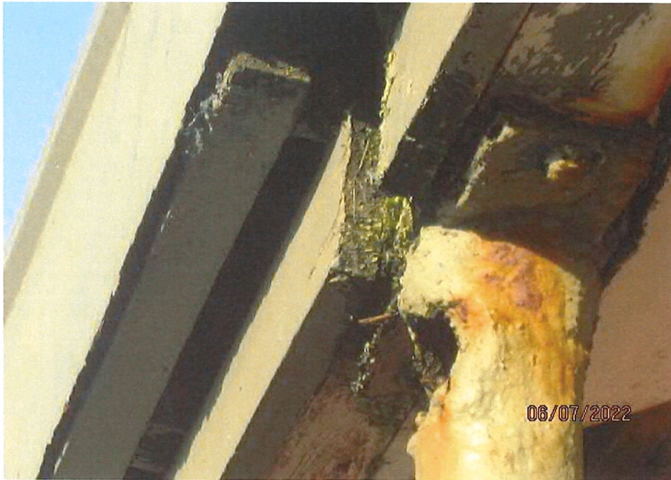
Typical view of veranda post heavily corroded and in very poor condition and the supported beam above
