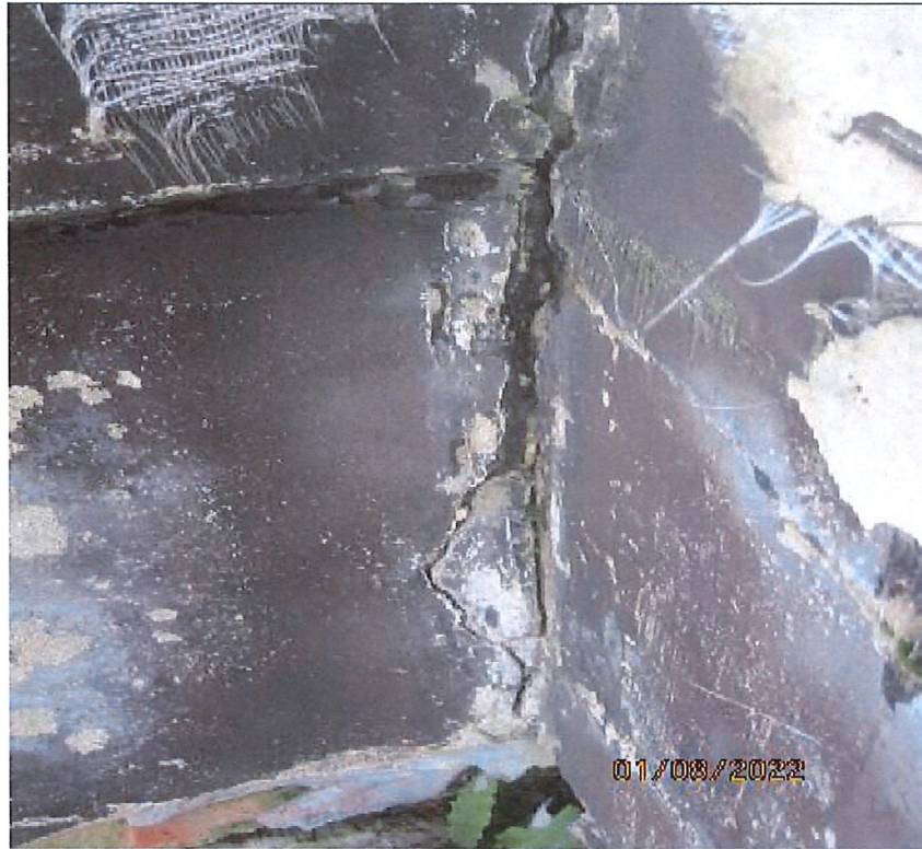
Large open cracks (15mm) extending deep into the walls supporting façade . Vegetation growing out of lower crack level
