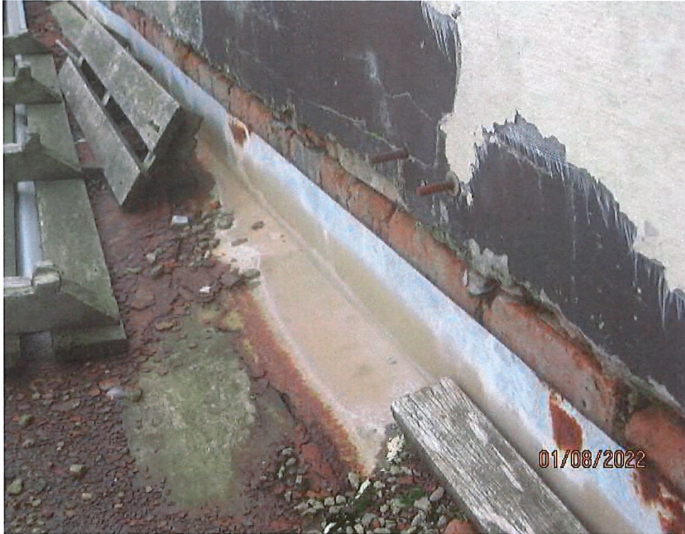
Typical condition of gutter behind façade, gutter rusted out, no over flashings to wall , deep recess extending into brick layer from missing overflashing allowing water inside the wall
