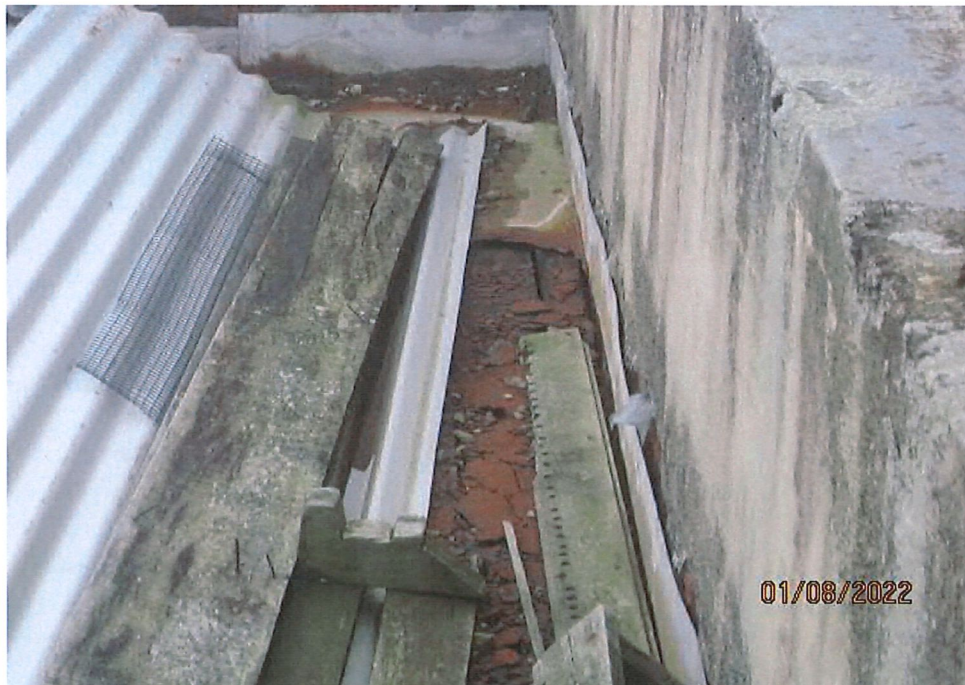
Typical condition to north end of gutter with rusted out gutter the supporting timber framing of gutter is all rotten. Open edge to upstand edge of gutter allowing water to track down behind upstand into the building
