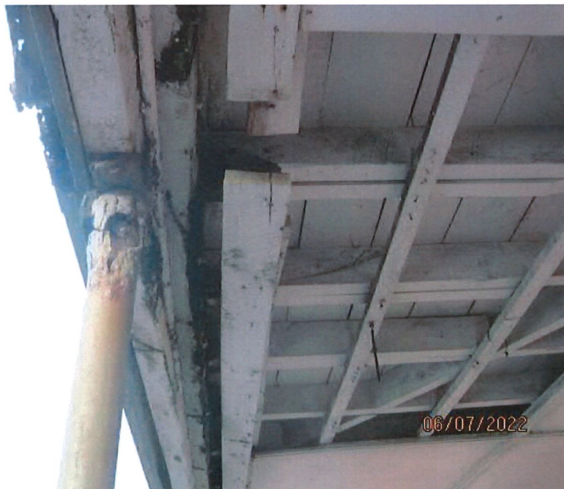
Top of post has disintegrated, and the outer beam is carrying most of the load to adjacent posts. The rafter to beam nail fixings have all withdrawn from the timber. Connection to this area of roof is very poor and on the verge of collapse.
