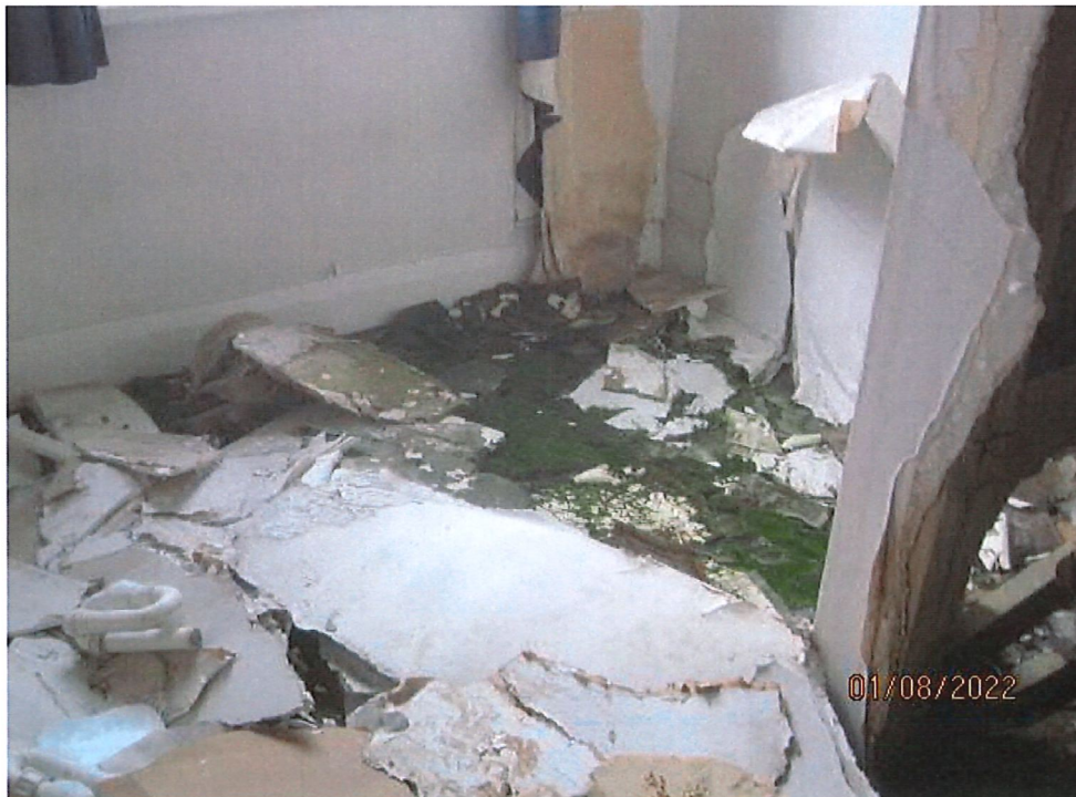
Typical damage to wall linings and the floor covered in moss from saturated flooring from water entering above. Condition of flooring and joists is likely to be deteriorated due to the saturated timber
