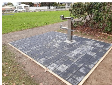
Accessible drinking water fountain including a bottle filler
