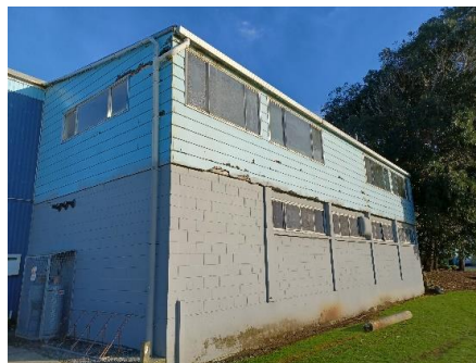
Older style clubrooms with deferred maintenance
