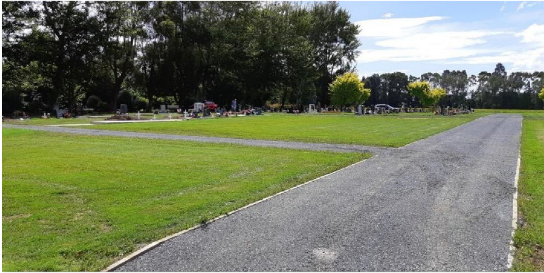
Figure 1: Work has been completed on improving access and drainage in Block 53. Bollards are to be installed to restrict vehicle access to the paths.
