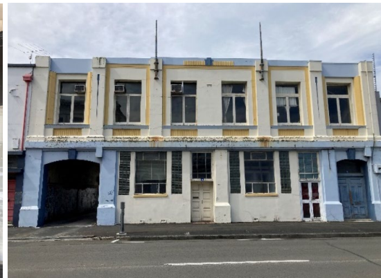
Deteriorating building. Lowe St
