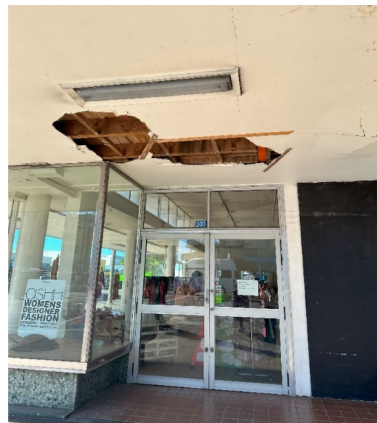
Main Street building decay. Gladstone Rd
