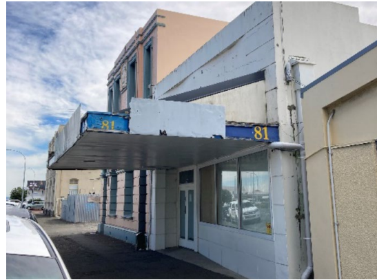
Deteriorating building. Childers Rd
