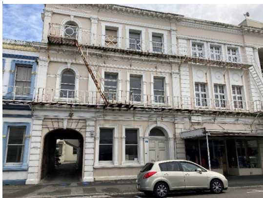
Masonic Hotel decaying façade. Lowe St
